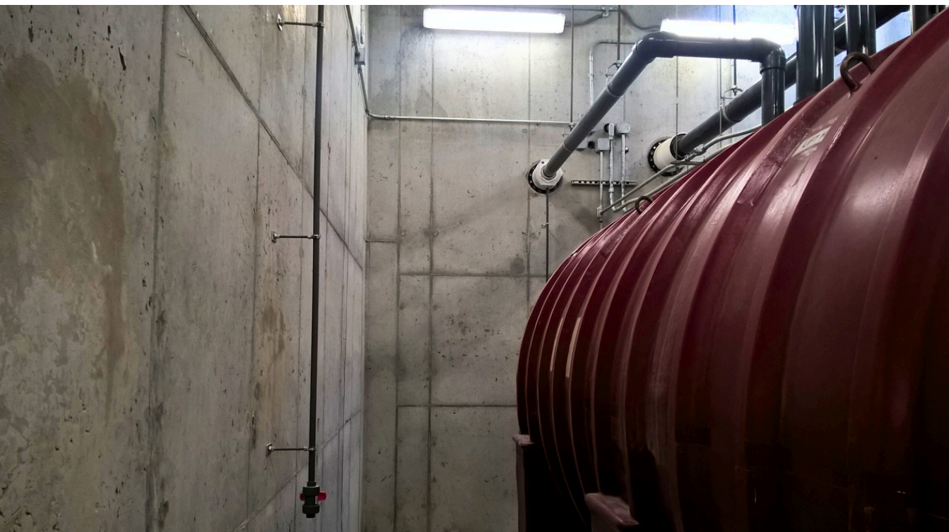
CANAL ROAD CHEMICAL WASTE STORAGE TANK REPLACEMENT Franklin Township, Somerset County, NJ
