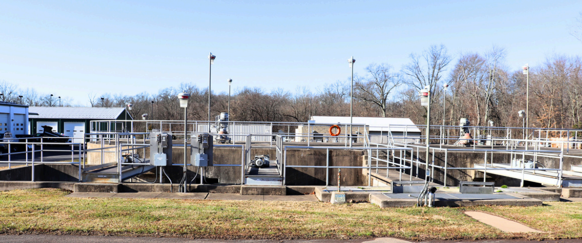
HARVEY AVENUE WASTEWATER TREATMENT PLANT Doylestown Township, Bucks County, PA
