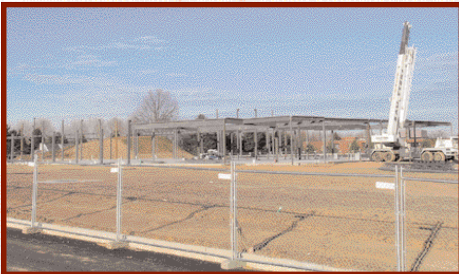
Steel for the new Horsham Library reaches toward the winter sky near the intersection of Babylon and Jarrett Roads. The contractor is Nason and Cullen Inc., King of Prussia, Pa. Completion is scheduled for Summer 2004.
